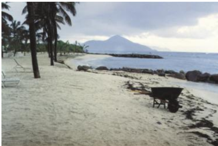
Groyne at Nisbett Plantation, Nevis. The sand has built up on the updrift side of the groyne in the foreground, while the waves reach further inland on the downdrift side as a result of erosion.
